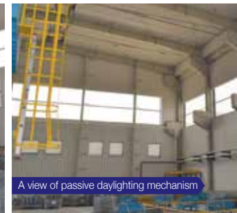
A view of passive daylighting mechanism
