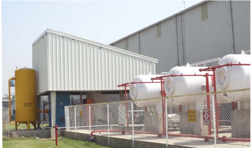
SNG Plant at Sheikhpura factory
